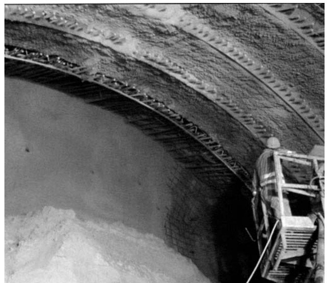
Figure 1. Spiles installed through the lattice girder to the face in every excavation step.
