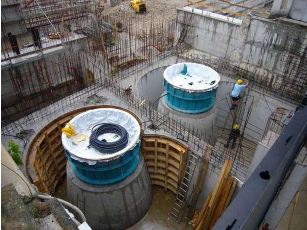
Figure 19: The two Kaplan machines
