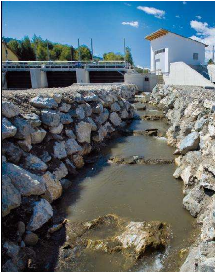
Figure 33: View of the power plant and fish ladder at Niklasdorf (BEA Electrics)
