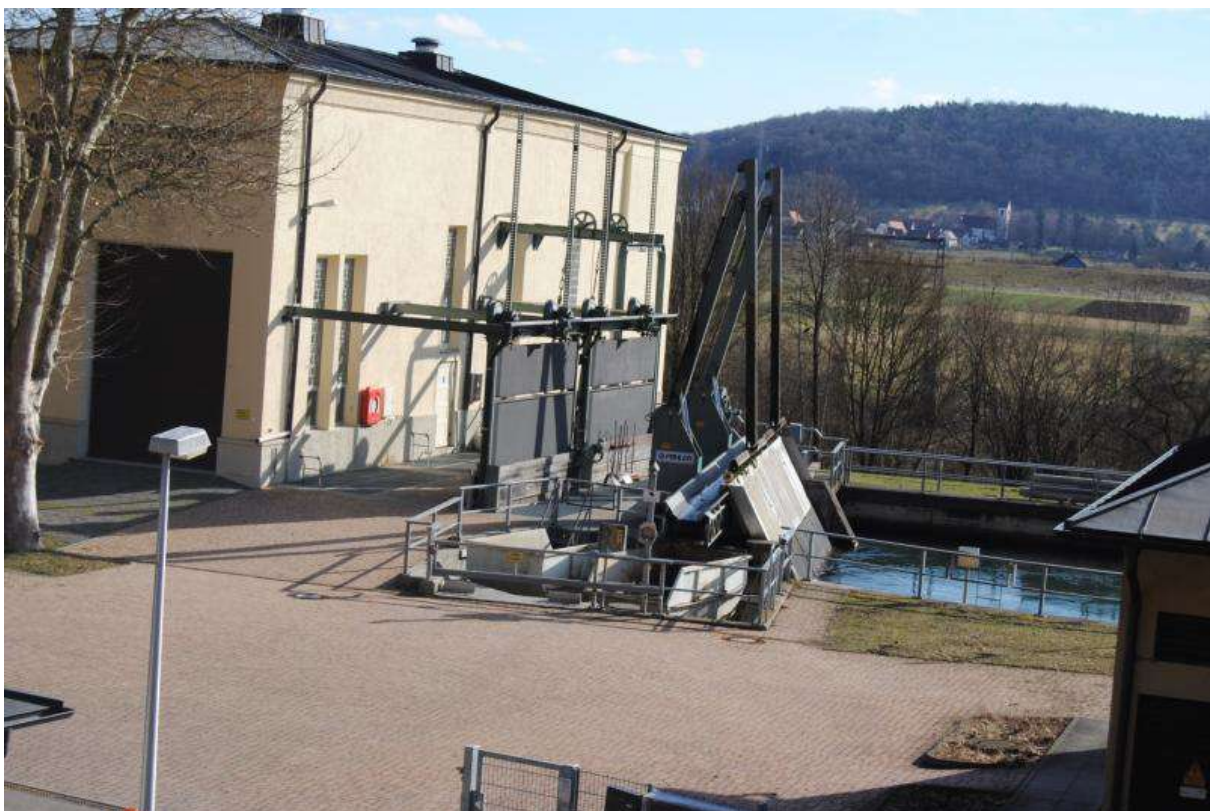
Figure 39: Trash rack clearing facility of main power house (photo [Renz, 2011])
