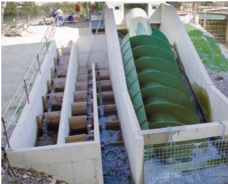
Figure 32: View of the MIF power plant in Kindberg (BEA Electrics)
