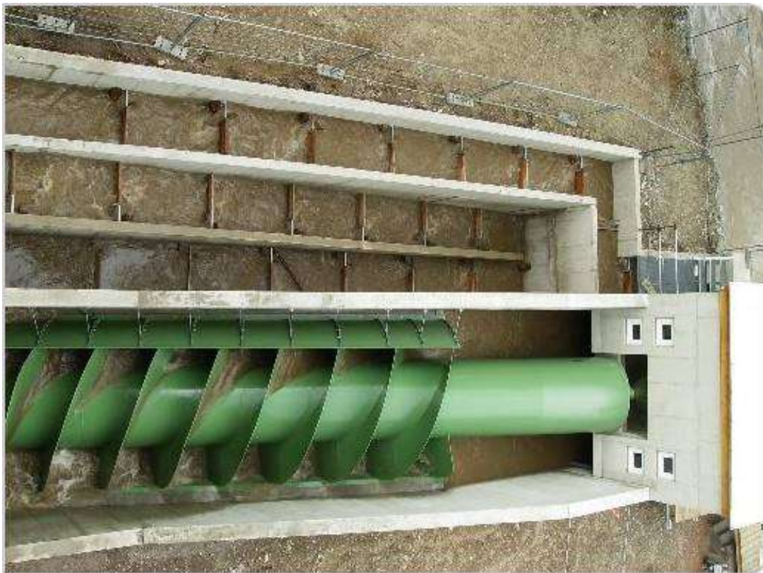
Figure 30: View from above of the MIF plant at Kindberg (Schalungsbau Hager Ges.m.b.H.)
